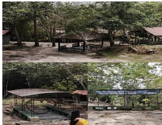
Figure 12. Damaged and unmaintained facilities in one of the tourist attractions in sei gohong Source: Researcher's documentation (2026)
